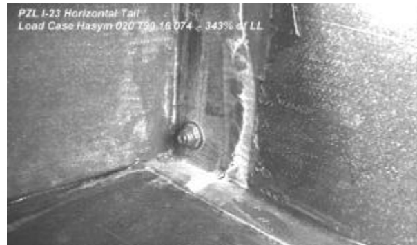
Fig. 9 Enlarged failure zone nearby rib 1R. In center is showed self-locking nut of the fitting.
